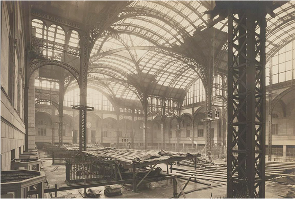
Penn Station under construction. (Avery Architectural and Fine Arts Library, Columbia University)
