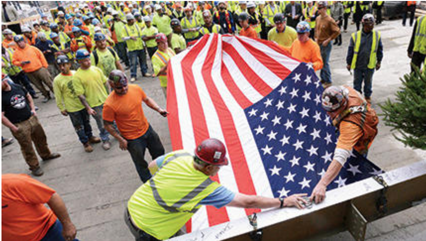
Construction workers prepare the final beam for placement atop the Lenfest Center for the Arts. Photo: Eileen Barroso
