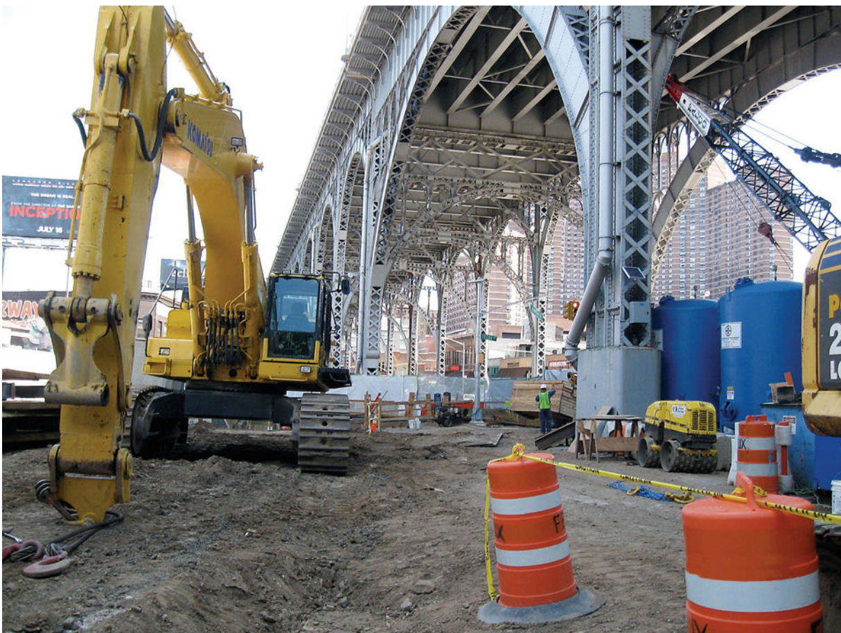
Columbia construction on 12th Avenue, beneath the Riverside Drive Viaduct. (Columbia Facilities)
