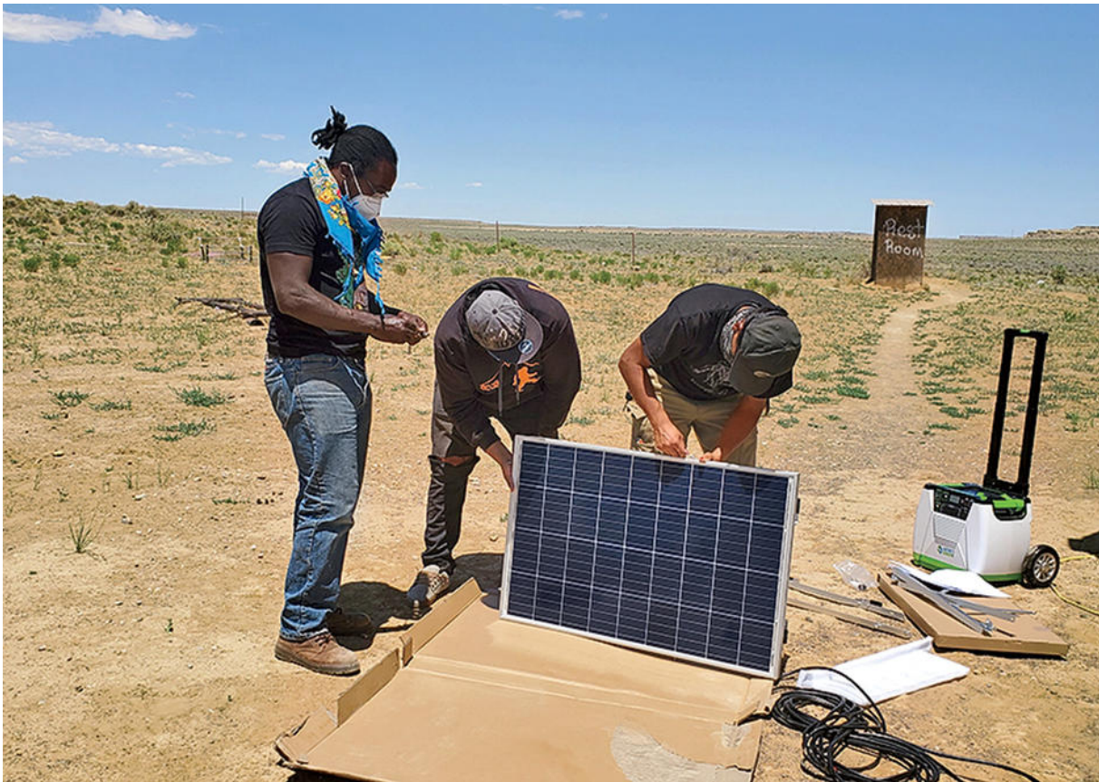
Collymore (left) installs solar generators on a family farm that doesn't have electricity.
