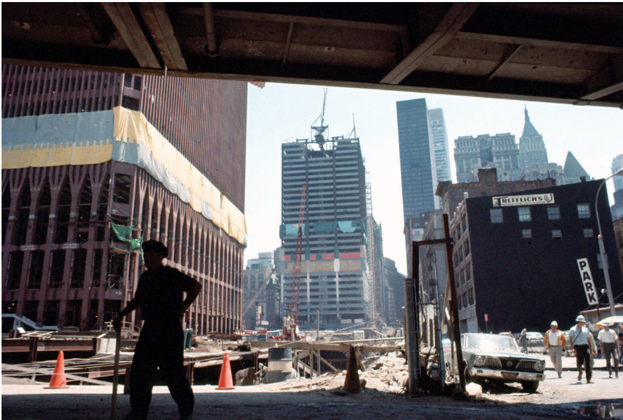
World Trade Center under construction, seen from West Street, Manhattan, 1970. (Camilo José Vergara)
