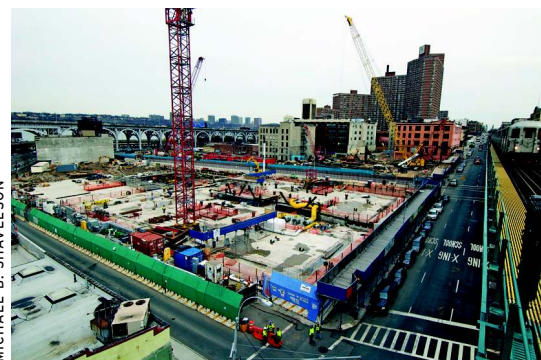
The site of Columbia’s future Manhattanville campus, pictured on March 18, facing northwest.
