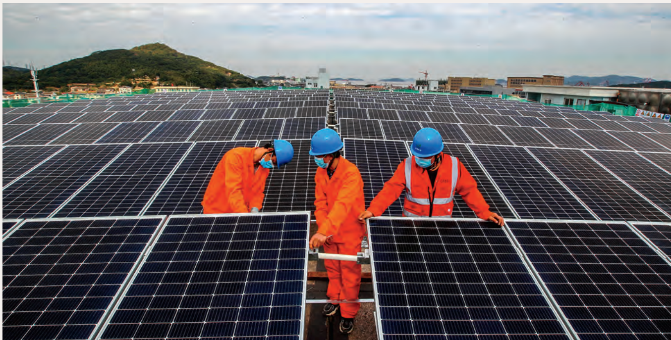
Workers install solar panels on the roof of a fish-processing plant in Zhoushan, China.
